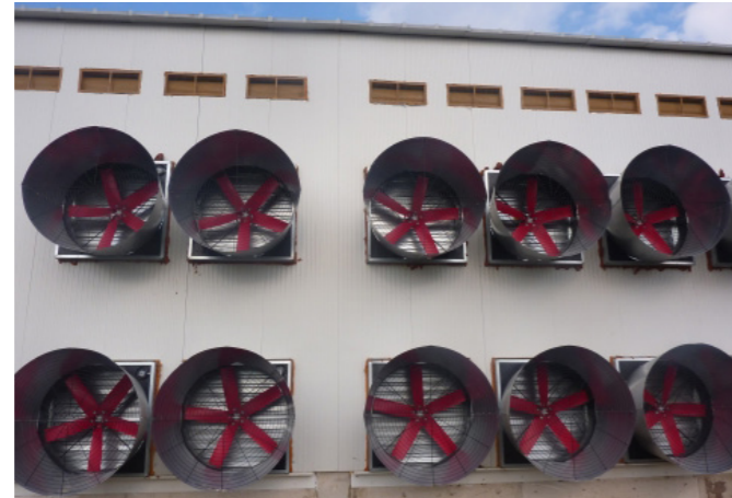
Ventilation applied in poultry houses in the Middle East
